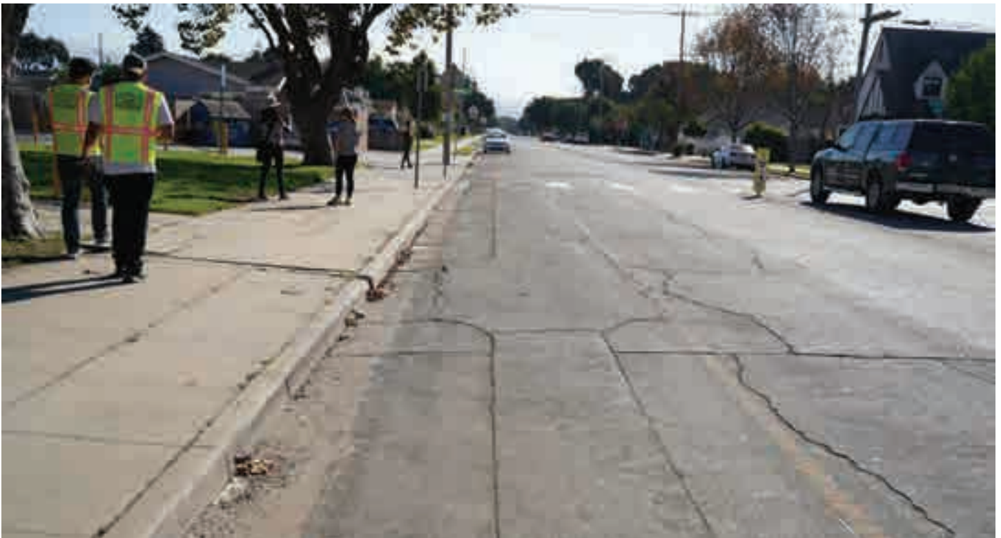
Widening the sidewalk to create a shared-use path is recommended for California St
