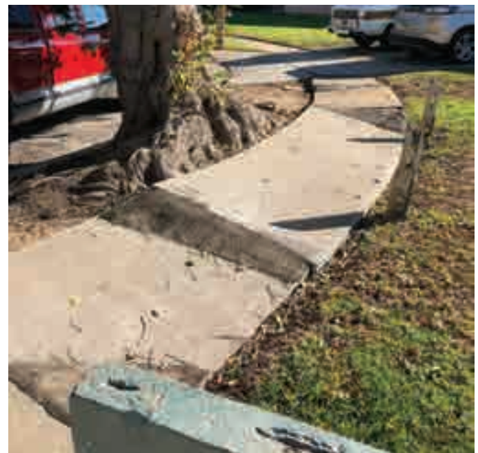
Broken sidewalk on Compton Way
