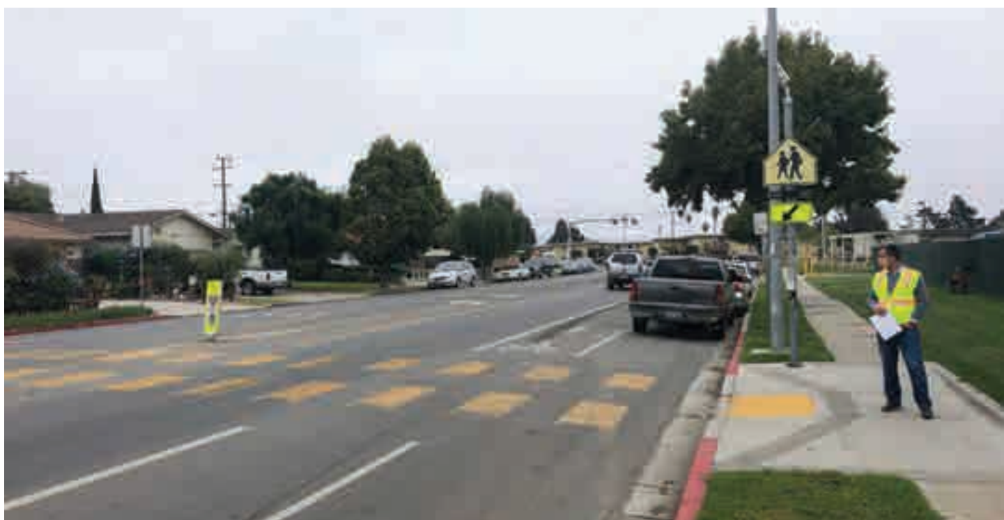
A road diet, bike lanes, and rectangular rapid flashing beacons were installed on John St
